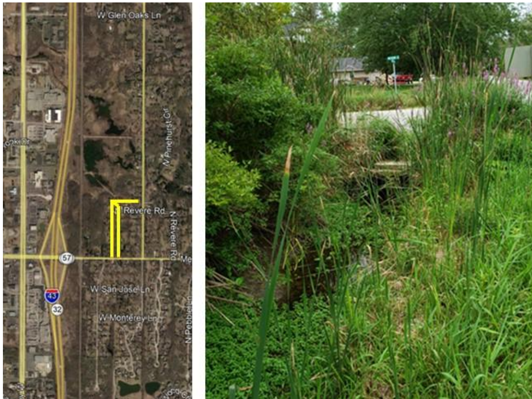
Figure 4. Map of study area showing location of proposed ditch modifications (left). Photograph of the existing ditch and culvert looking south towards Revere Road and Prairie View Lane intersection (right).
