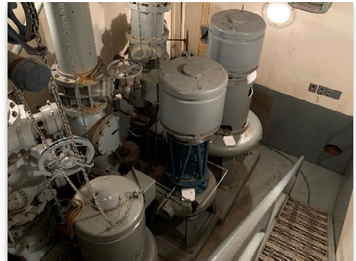
Existing dry pit pumps
