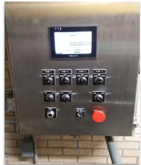
Existing LS E control panel
