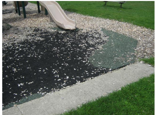
Aging safety surfacing at north playground
