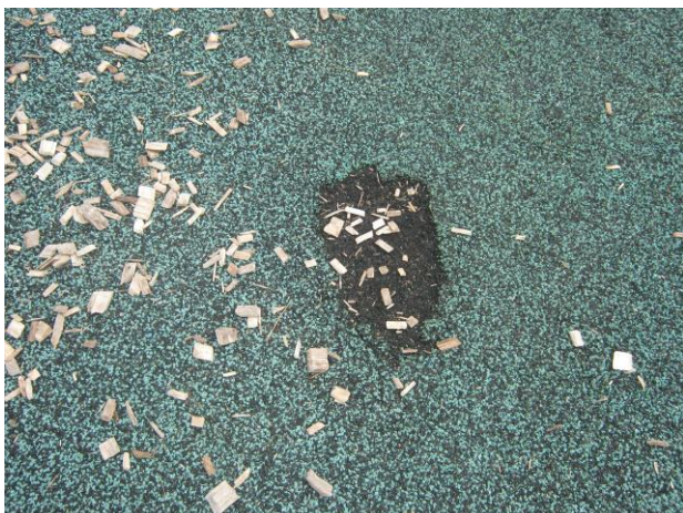
Worn areas in playground surfacing
