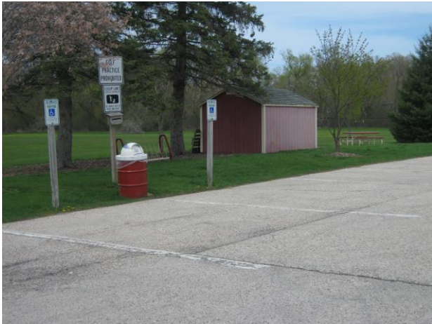
No ADA parking pavement marking
