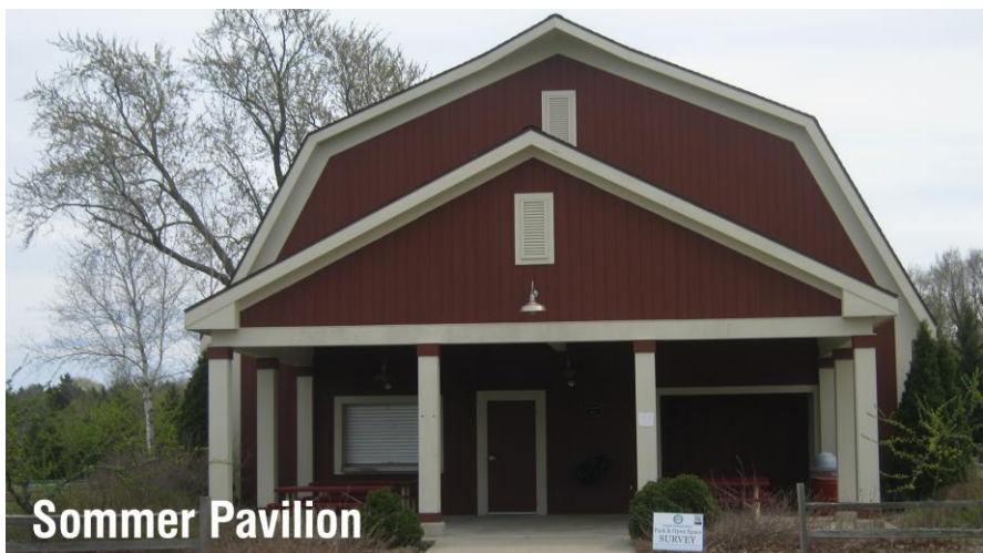
Worn safety surfacing
